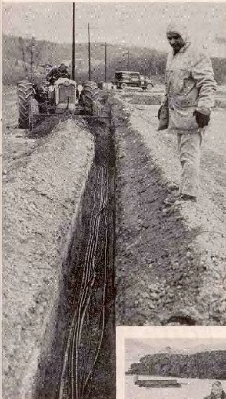
Above: Laying cable to interlocker is made a simpler operation, thanks to remarkable machine. As Signalman G. H. Webster operates tractor (Fordson Trench Hog) and Signal Foreman J. J. Hacker, right , helps direct operation, machine "back fills" over cable laid by signal department employees. The same tractor, using a different attachment, had earlier dug trench it is now filling. Devices such as this have cut down on much heavy work which was once performed manually; are saving manpower for special-skill duties.
