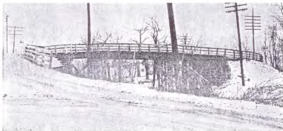
ANOTHER danger spot is the wooden bridge over the L & N tracks on the Walton-Nicholson Pike. It has been the scene of numerous accidents, including several fatalities.
