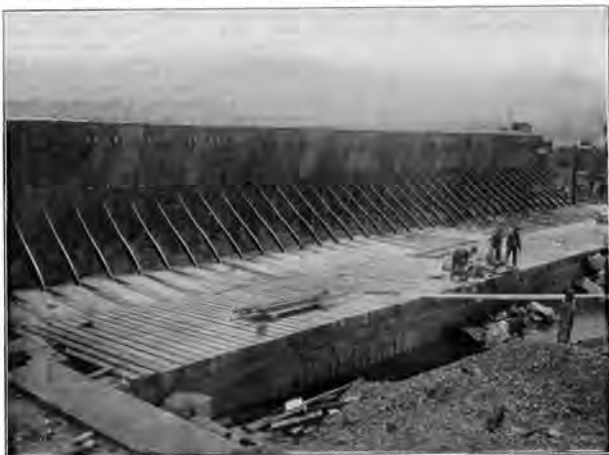
FIG. 5. CHANOINE WICKETS IN RAISED POSITION (WITHIN COFFERDAM) AT DAM NO. 4, OHIO RIVER.
