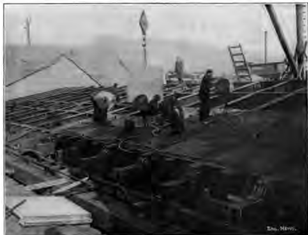
FIG. 8. CONSTRUCTION OF THE STEEL LEAF OF THE BEARTRAP AT DAM NO. 3, OHIO RIVER.
