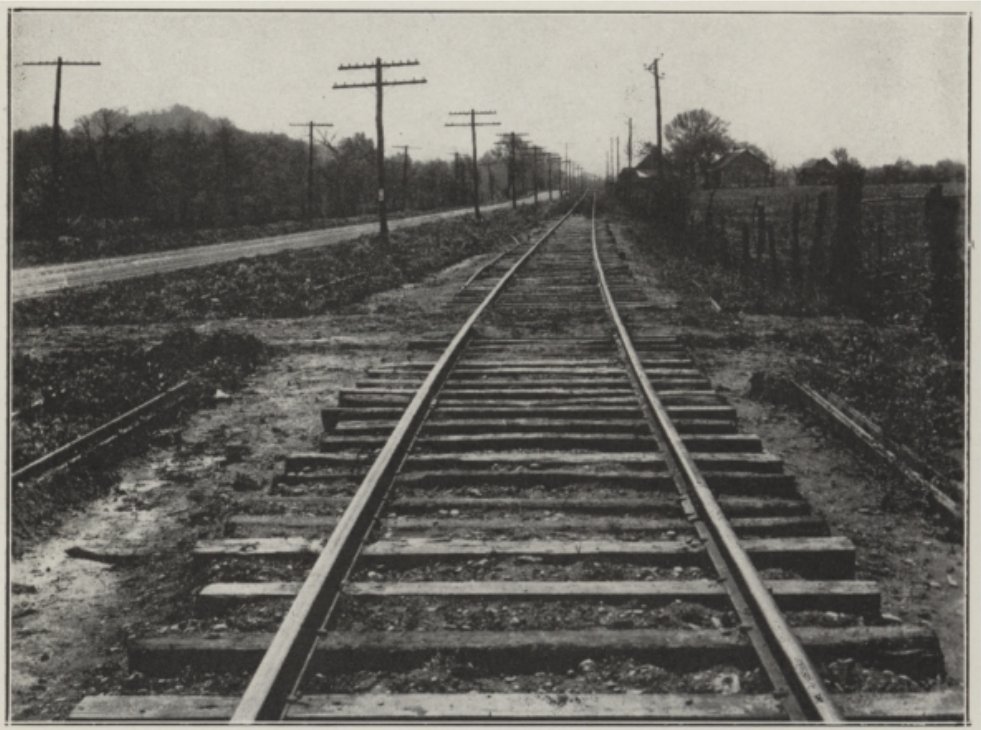
A section of the C. & W. R. R. immediately after the sale in 1927. Looking toward Worthville, new rail being laid.
