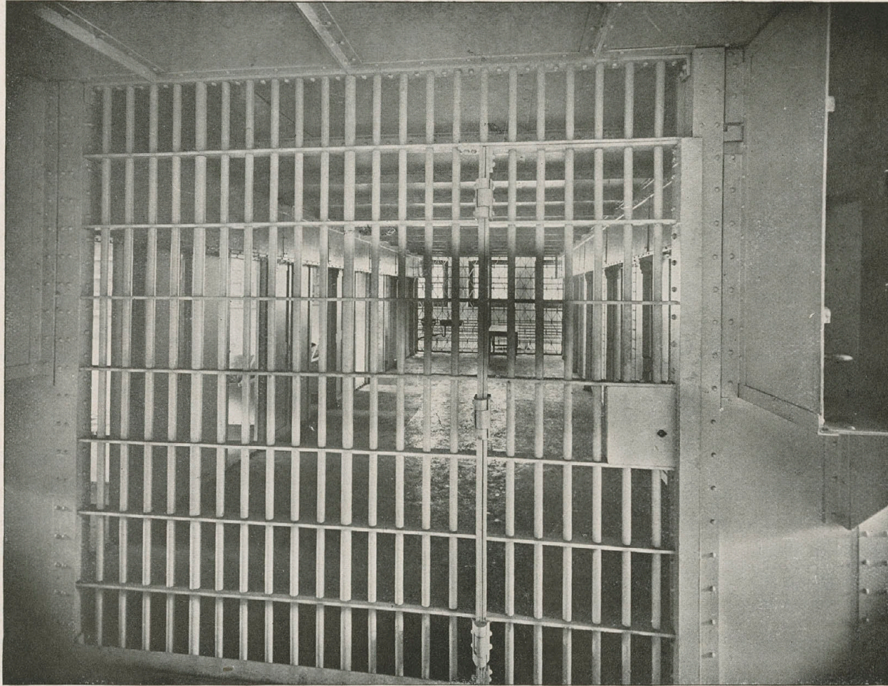
Interior View through Central Prisoners' Corridor, showing Our Tool Proof Cells and Patent Sliding Cell Doors in the New Jail at Newport, Ky.
